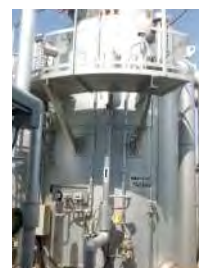
Remaining heat boiler
