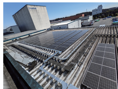
Solar Panel at Tsukuba Plant
